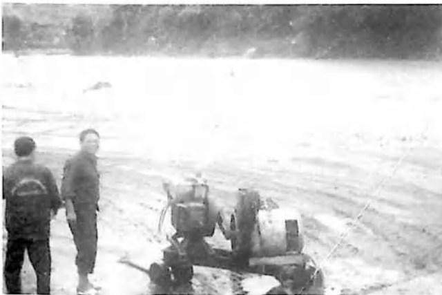
Workers are making preparations for building a temporary bridge on a bvnoss
